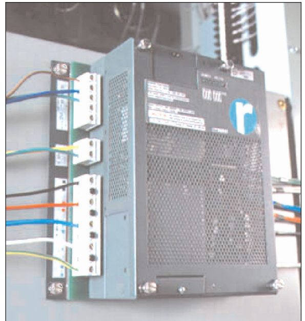
Figure 4. The Reliable Power Meters Multipoint Power Recorder shown installed in a switchboard as part of a power-quality monitoring network at a data center for a major bank.
